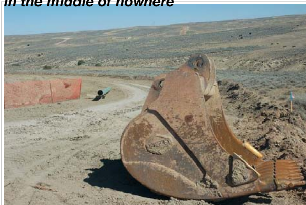
Earth-moving equipment in the foreground and pipe in the background are testament to the work going on at the Fortification Creek site. Two coal-bed methane companies are moving forward with plans to tap into what is believed to be a massive store of methane which would produce natural gas, a vital energy source for America.
