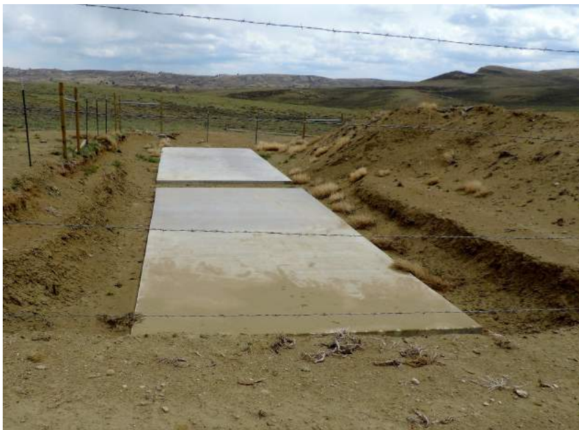
Two concrete pads were the extent of construction at the DKRW site.
