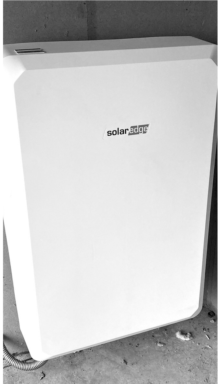
An example of a solar battery installation. Photo courtesy of Creative Energies.
